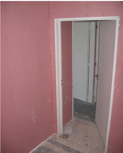
DATA CENTER FROM INSIDE - DRY WALLS - RED GYPSUM BOARDS (FIRE RESISTANT)
