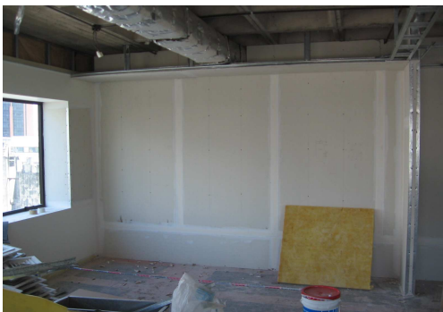
MEETING ROOM FROM INSIDE - DRY WALLS - DOUBLE GYPSUM BOARD FOR ACOUSTIC INSULATION
